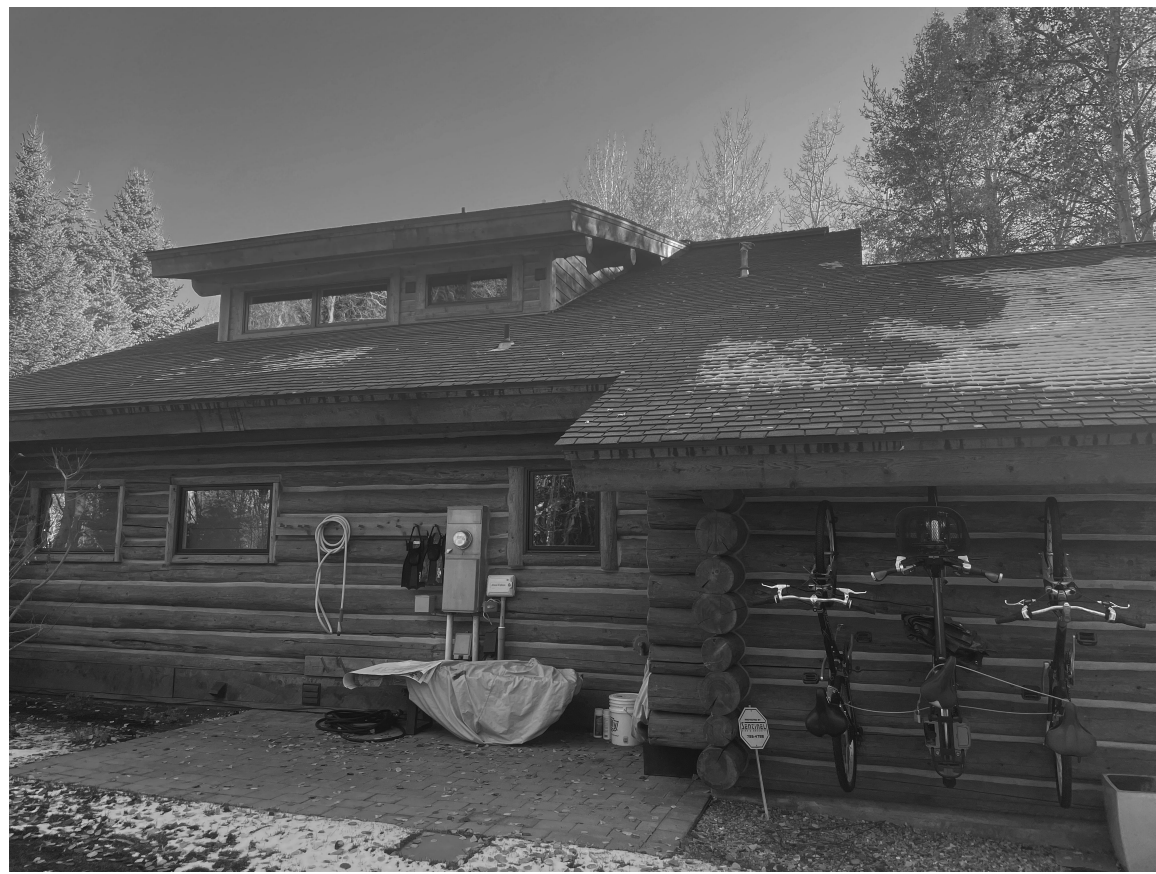
PHOTO #5 -ELEC METER TO BE RELOCATED AND STORAGE AREA RO BE REMOVED
